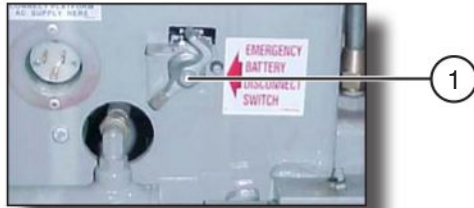
Figure 2-1. Main Power Disconnect Switch
